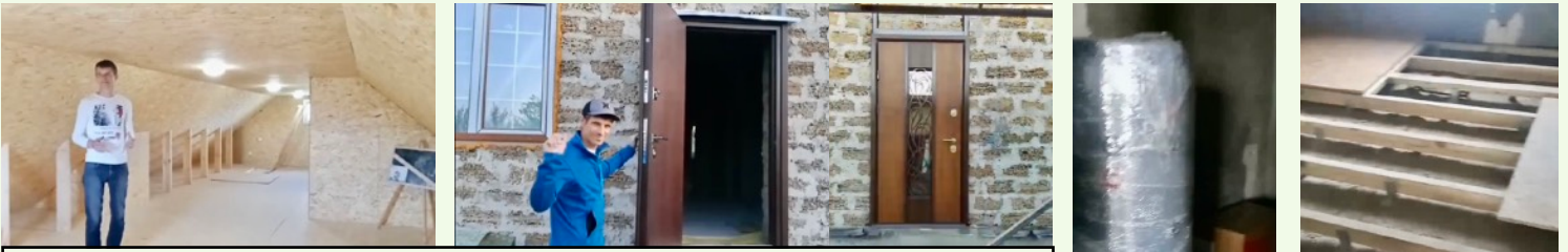
By the grace of God, during the COVID season, RLM & DHF have been providing funds for the interior of the building project of the Children's Home in Kremenchuk. To date, the attic was finished (L) and two security doors (M) and the water heater (R) have been installed.
